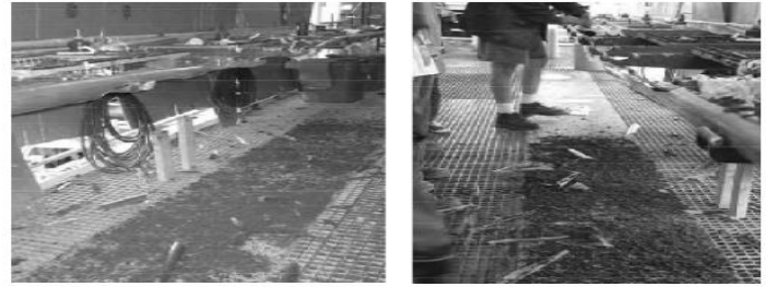
Figure 43: (a) Burst pipes on hydrate formation (b) Eliminating clogging in pipes [33]
